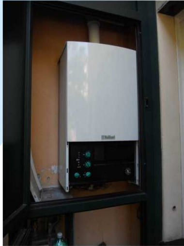
LOW BOILER EFFICIENCY
