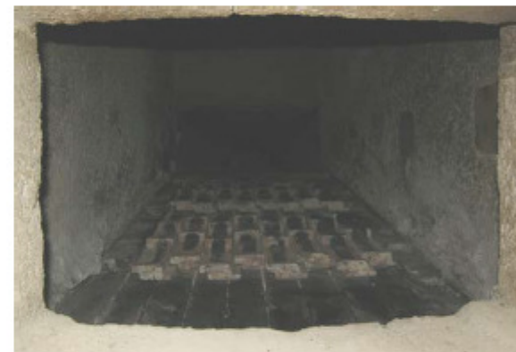
Furnace C: Stepping Grate
